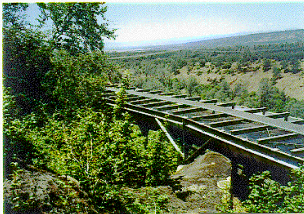
Photograph 6. - South Canal: Type #132 metal flume identical to South Canal installations (Eagle Canyon Canal flume shown).
