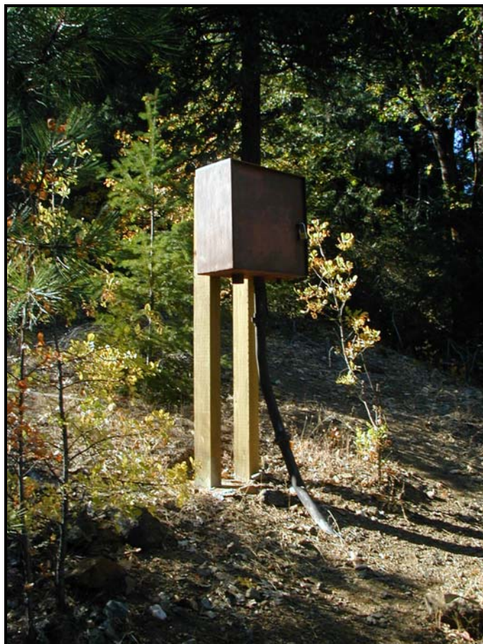
Steel gage house mounted to 4x6 posts in concrete: South Fork Trinity at Forest Glen.
